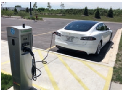
Electric car charging point at the new headquarters building for Renishaw, Inc.
